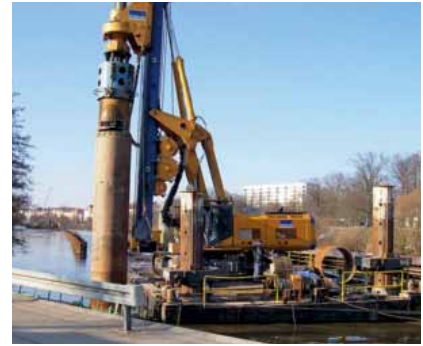
Drilling and piling equipment on a construction site: a robust and reliable machine controller is required.
