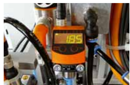
Pressure measurement in pneumatic systems.
