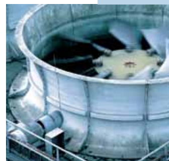
Coolant towers and exhaust fans.
