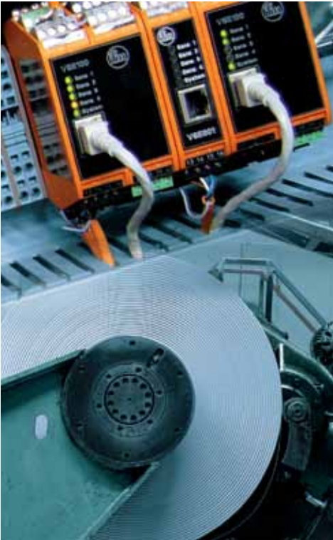
Online condition monitoring
